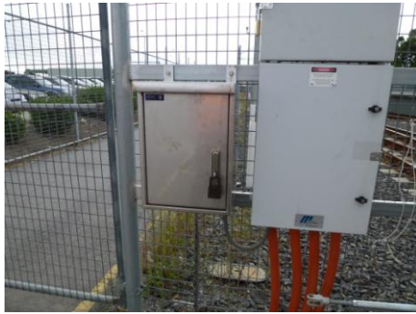
Cabinet next to the gate control box
