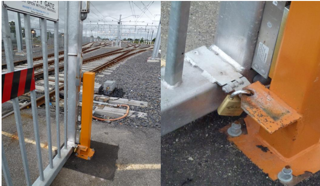
Gates secured “open” by the latch and padlocks provided.
